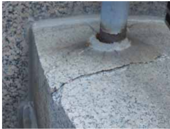
Fig. 2.1.A.9 Damage to low granite wall enclosing the window well.
