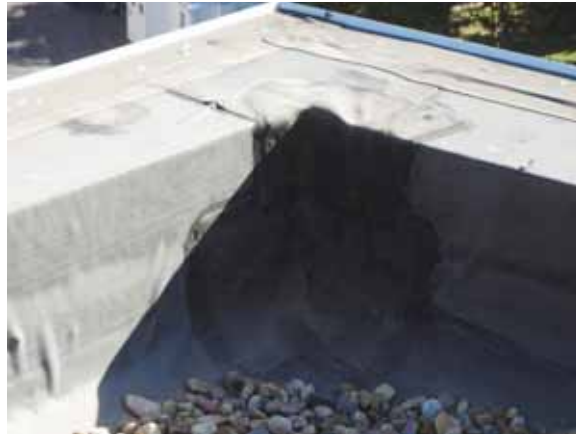
Fig. 2.1.A.18 Repairs to roof membrane and bubbling of roof membrane.
