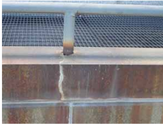
Fig. 2.1.A.8 Damage and staining to low granite wall enclosing the window well from corroded low pipe railing.
