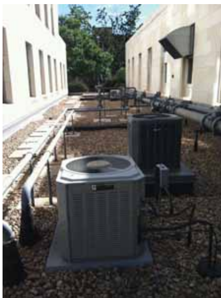
View of the ballasted grade-level roof over the basement of the Power Plant Building and adjacent to the Capitol Annex Building, looking east from the west side of the roof
