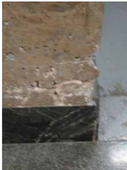
Fig. 3.8.C.2 Damage to golden travertine marble in the Basement elevator lobby.
