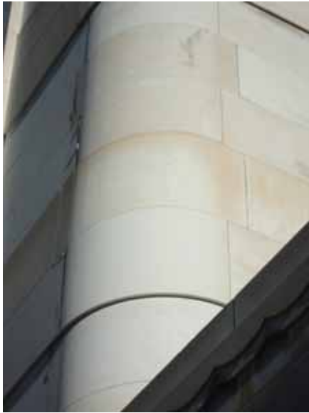
Fig. 2.1.A.6 Soiled rounded marble corner panels with joint deterioration.
