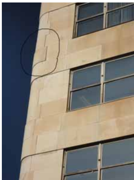
Fig. 2.1.A.2 Marble panels moving out of flush.
