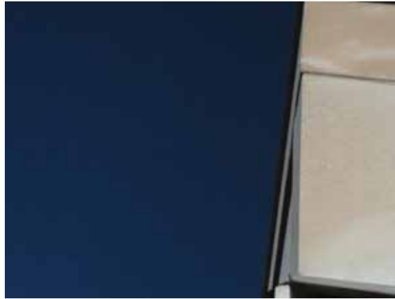
Fig. 2.1.A.3 Panels cladding the Penthouse are in generally poor condition.
