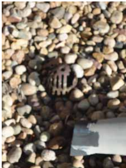
Fig. 2.1.A.17 Corroded drain cover, south roof at grade level.
