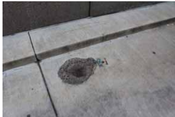
Figure 2.3.A.9 – Broken Site Concrete, Recommended for Replacement
