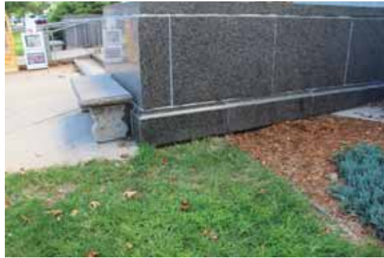
Figure 2.3.A.5 – Marble Site Wall Settling
