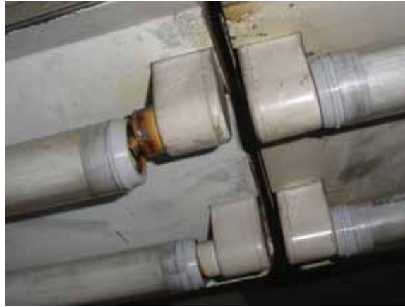
Fig. 2.4.B.1 - Broken bulb hanging
