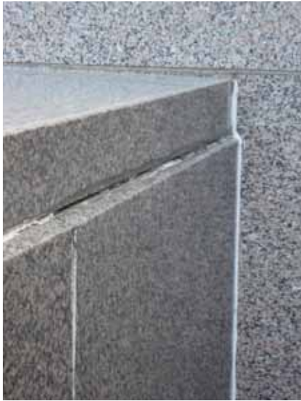
Fig. 2.1.A.11 Deteriorating sealant between granite panels.
