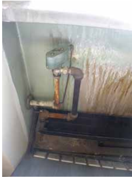
Fig. 2.4.A.13 - Pneumatic Control Valve (Convector)
