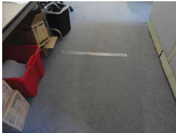
Fig. 3.7.C.5 Taped carpet seam creating a tripping hazard.
