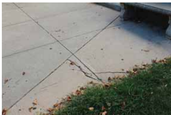
Figure 2.3.A.7 – Site Concrete Crack
