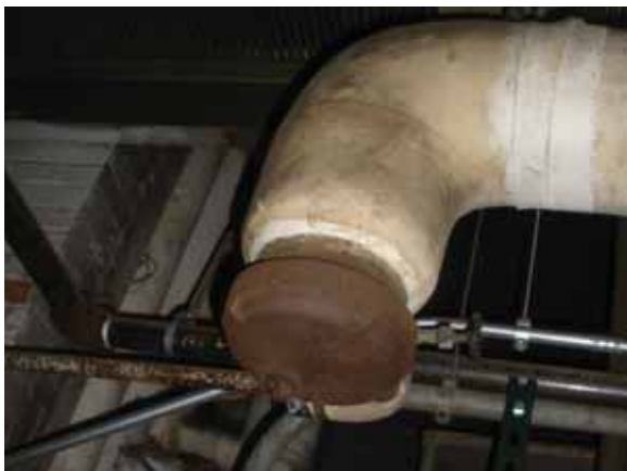
Fig. 2.4.A.6 - Abandoned Steam Pipe
