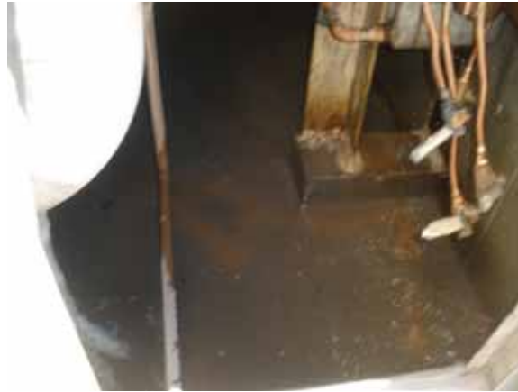
Fig. 2.4.A.7 – Standing water in AHU Cooling Coil Drain Pan
