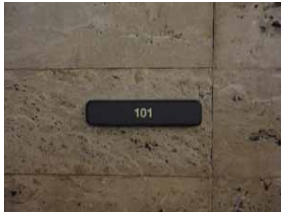
Fig. 3.1.C.3 Grout missing in joints between golden travertine marble panels noted throughout.
