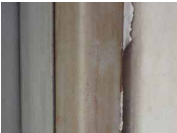
Fig. 2.1.A.15 Deteriorating sealant surrounding window frames.
