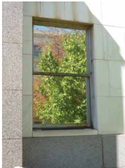
Zone 1 Exterior Facade: Typical window with some rusting and peeling paint
