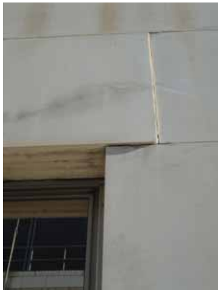
Fig. 2.1.A.1 Marble panel cracking/ moving out of flush.
