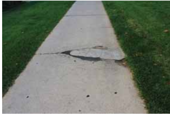
Figure 2.3.A.8 – Site Concrete Patch, Recommended for Replacement
