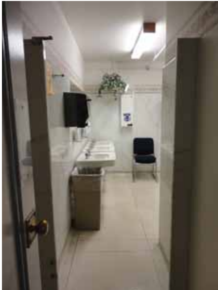
Fig. 2.1.C.5 Wall panels protruding into accessible entry space of the restroom.
