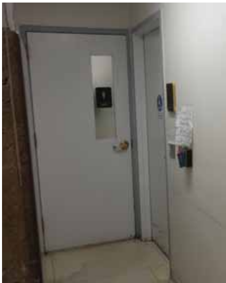
Fig. 2.1.C.6 Unisex Restroom at the Basement Level with broken automatic door opener and with accessible entry space infringed upon by the nearby Men's Restroom door which swings out into the space.
