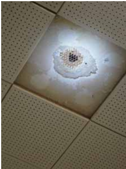
Fig. 3.1.C.1 One-foot square perforated ceiling tiles glued to the plaster ceiling in poor condition.
