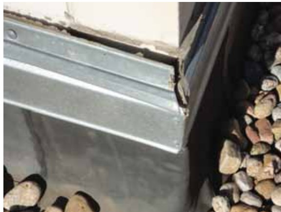
Fig. 2.1.A.19 Flashing pulling away from the Penthouse wall.
