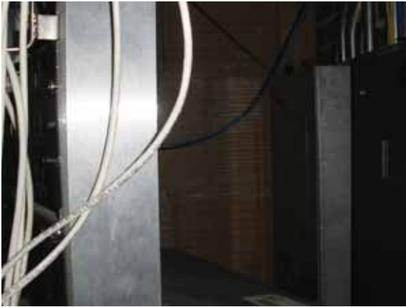
Fig. 2.4.B.4 - Panel not accessible
