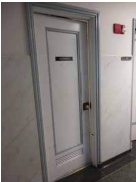
Fig. 2.1.C.1 Knob-style door handle on restroom door with no automatic door opener.
