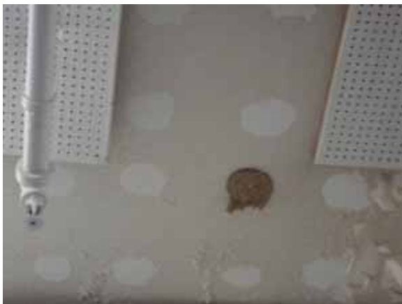
Fig. 3.1.C.2 One-foot square perforated ceiling tiles glued to the plaster ceiling in poor condition.
