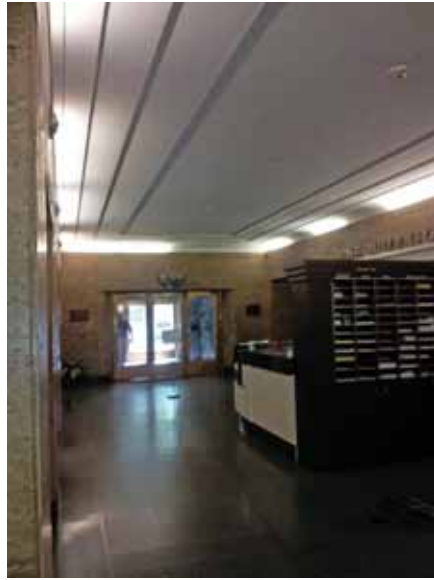
Zone 2 Interior Lobbies and Circulation: First floor central lobby with terrazzo flooring, marble wall panels and a shallow plaster coffer ceiling
