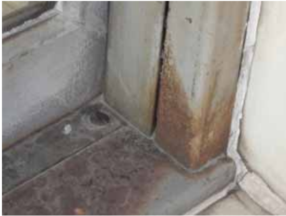
Fig. 2.1.A.13 Corroding metal window frame.
