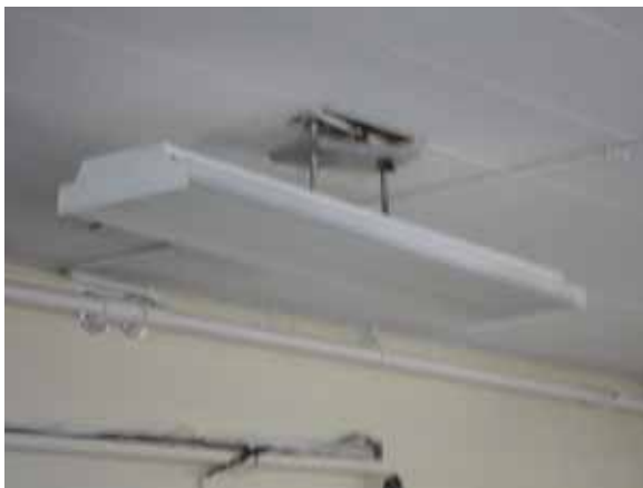
Fig. 3.7.C.2 Light fixture pulling loose from the ceiling.
