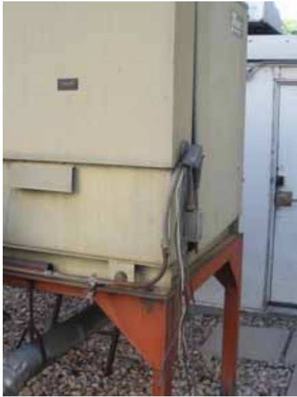
Fig. 2.4.A.4 - Abandoned Trane Chiller
