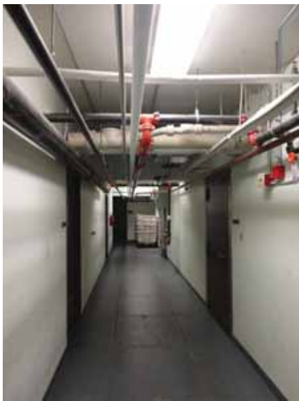
Fig. 3.9.C.1 Minor damage to the main service corridor walls and concrete floors.
