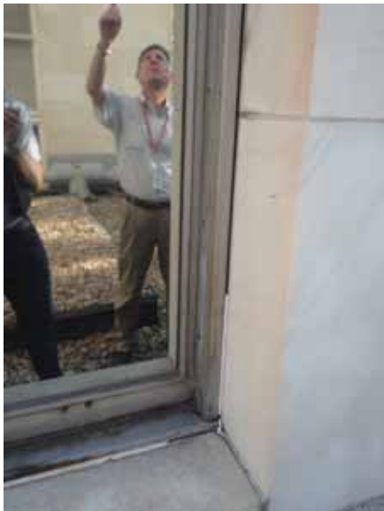
Fig. 2.1.A.14 Corroding metal window frame and deteriorating sealant.
