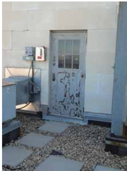
Fig. 2.1.A.16 Corroding door at the Penthouse Level.
