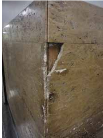
Fig. 3.8.C.1 Damage to golden travertine marble in the Basement elevator lobby.
