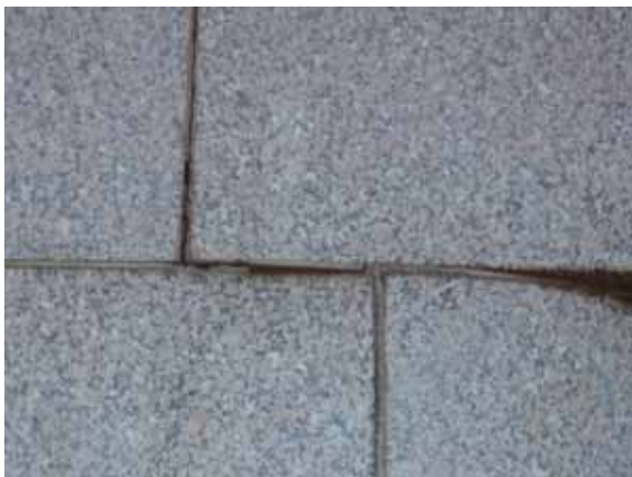
Fig. 2.1.A.7 Deteriorated sealant between granite panels.
