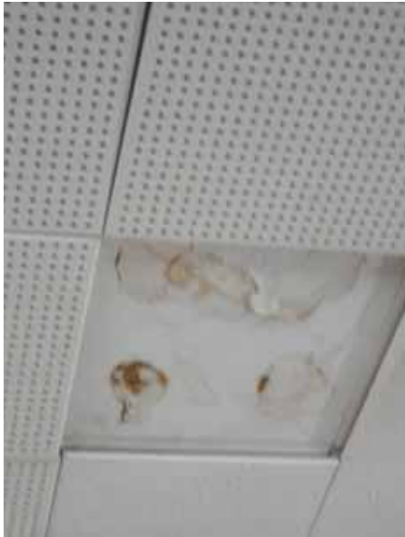
Fig. 3.7.C.1 One-foot square perforated ceiling tiles glued to the plaster ceiling in poor condition.
