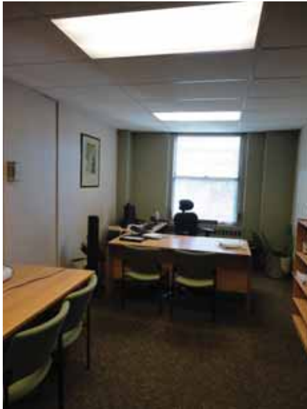
Fig. 3.3.C.1 Minor sagging of 2x4 acoustic ceiling tiles in an office.
