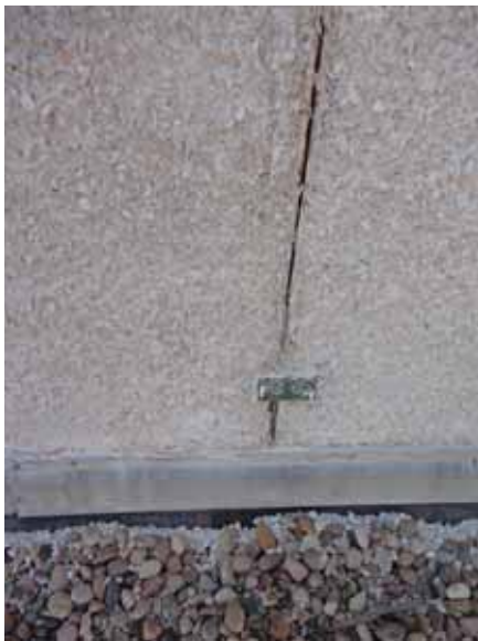
Fig. 2.1.A.9 Sealant failure at joints between precast aggregate panels.
