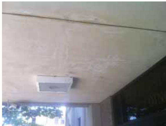
Fig. 2.1.A.16 Water damage observed under the east Sherman Street Entrance canopy.
