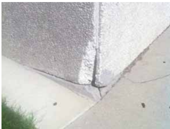
Fig. 2.1.A.1 Spalling at an exterior corner of the building.
