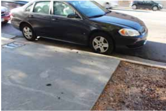
Figure 2.3.A.10 Site Concrete Crack, Recommended for Replacement
