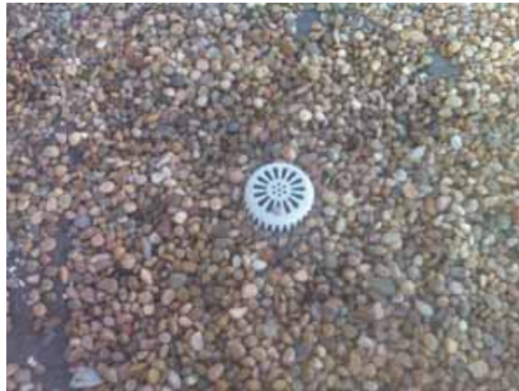
Fig. 2.1.A.12 Area where ballast is thin and roof membrane is exposed.
