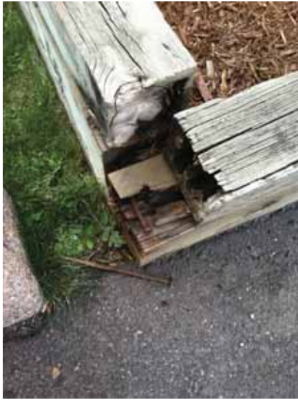
Fig. 2.1.A.17 Damaged railroad ties with exposed nails at raised landscaping bed along the east Sherman Street facade.
