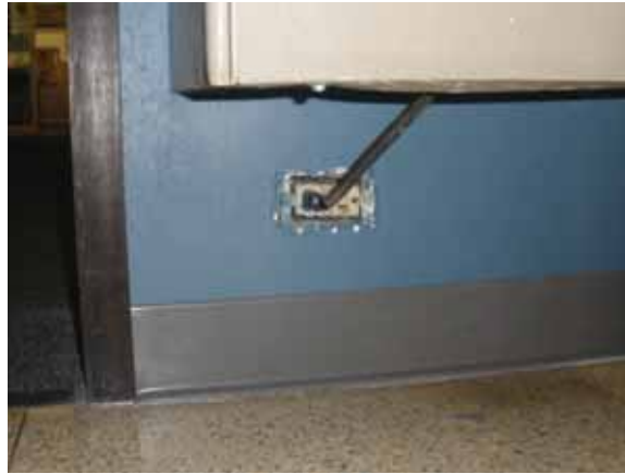
Fig. 2.4.A.7 - No cover on receptacle
