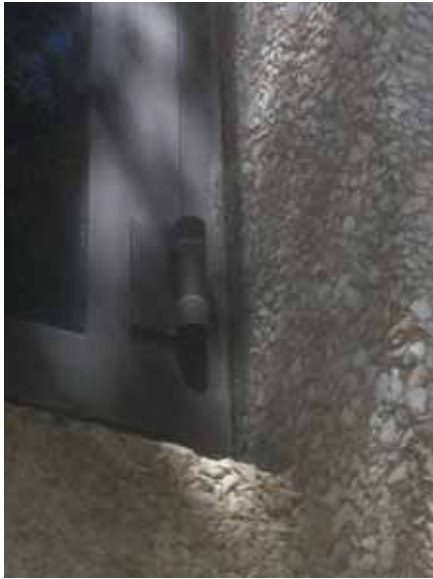
Fig. 2.1.A.11 Sealant failure around windows.
