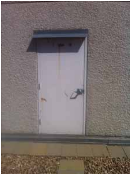
Fig. 2.1.A.15 Rusting door to the Penthouse.
