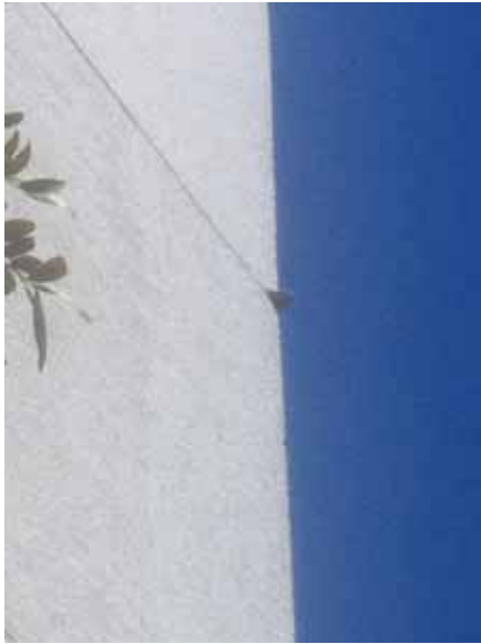
Fig. 2.1.A.3 Piece of aggregate lodged in the side of the building at the south-east corner.
