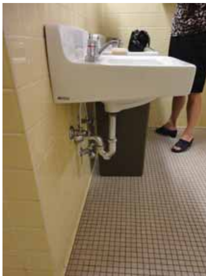
Fig. 2.1.C.1 Accessible lavatory without insulation wrapped around the pipes.
