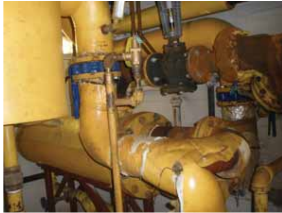
Fig. 2.4.A.14 - Steam / HW Heat Exchanger
