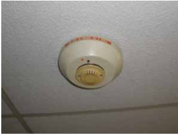
Fig. 2.4.A.5 - Old smoke detector
