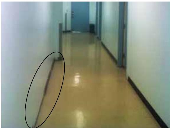
Fig. 3.9.C.1 Vinyl base molding cracking and peeling away from the wall.
