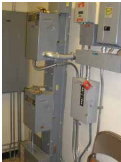
Fig. 2.4.A.1 - Bus duct in electrical rooms on each floor
