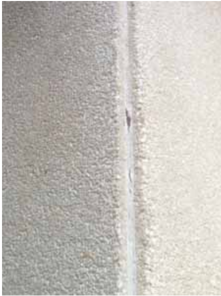
Fig. 2.1.A.8 Sealant failure at control joints.
