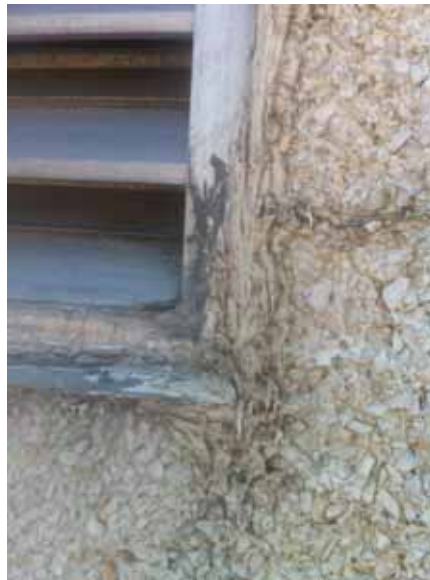
Fig. 2.1.A.6 Poor sealant repair and resulting staining of precast aggregate Penthouse panels.
