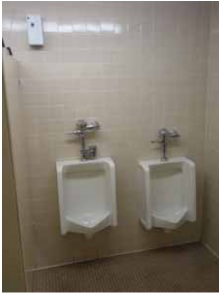
Fig. 3.1.C.2 Tile flooring in restrooms found to be dirty in some locations throughout the building.
