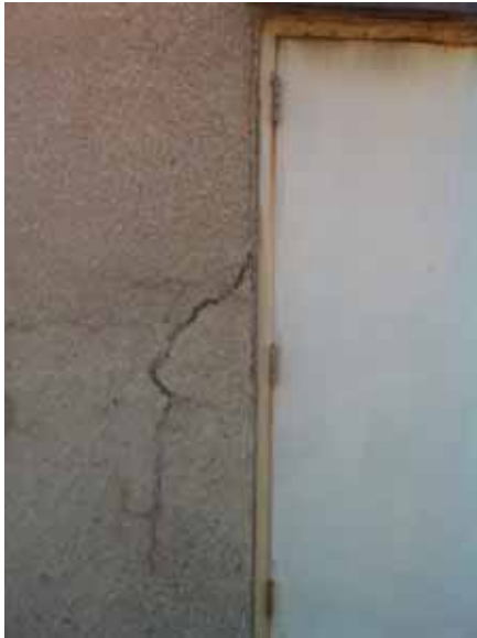
Fig. 2.1.A.14 Rusting door and door frame to the Penthouse and cracked precast panel.
