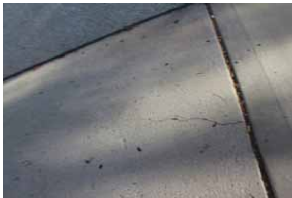
Figure 2.3.A.9 Site Concrete Crack
