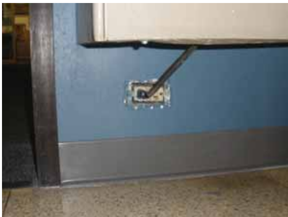
Fig. 2.4.B.2 - Receptacle missing cover
