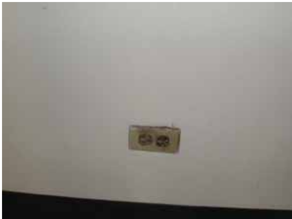
Fig. 2.4.A.6 - Burnt out receptacle
