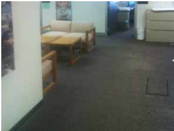
Fig. 3.2.C.1 Typical stained, dirty, and generally deteriorated carpet.
