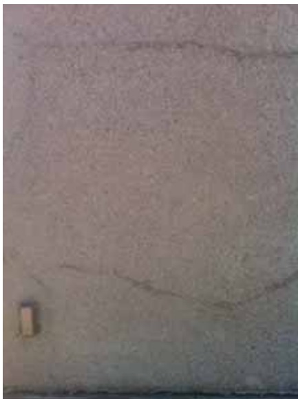
Fig. 2.1.A.4 Cracked panels, Penthouse Level.
