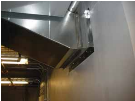
Fig. 2.4.A.12 - Elevator AC Unit Serving Electrical Room
